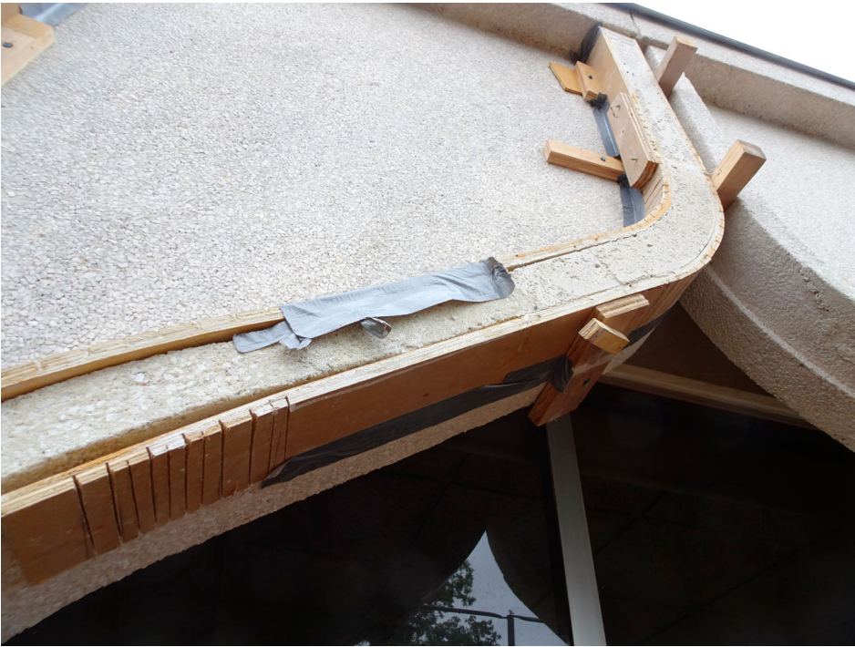
Figure 6. During the mock-ups, a process was developed for shaping the formwork around the curved contours of the concrete. (Photo courtesy of Mike Ford, AIA).
