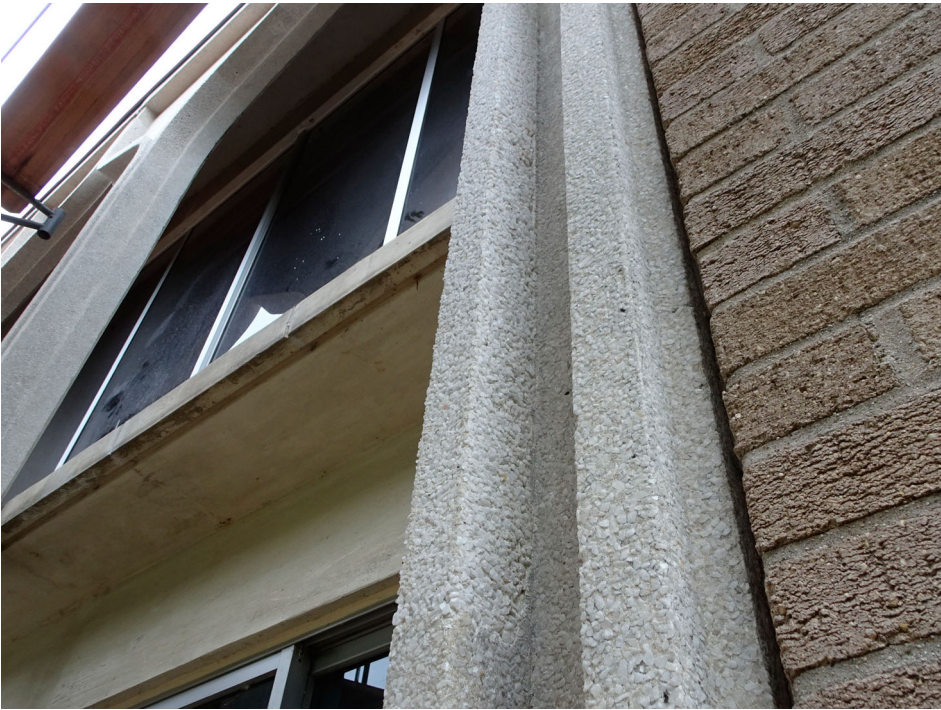
Figure 7. An example of the completed repairs at a window perimeter, showing the successful match of the repair to the original exposed aggregate precast concrete. (Photo courtesy of Mike Ford, AIA).
