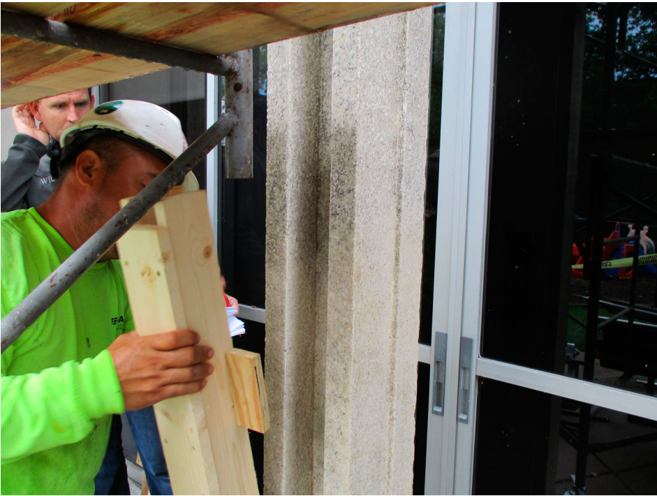
Figure 5. As part of the mock-ups, each step of the concrete repair process was evaluated, including the formwork and finishing techniques. (Photo courtesy of Paul Gaudette, FACI).
